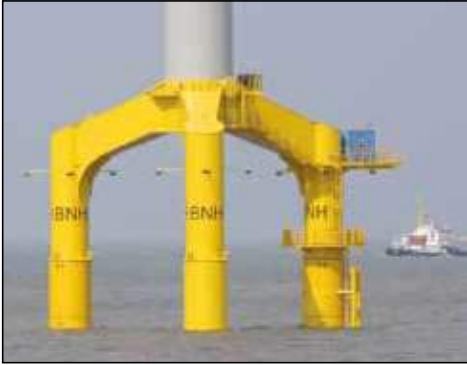
▲ Offshore wind turbines levelling: Enerpac's synchronous lifting system was the solution for levelling support cross pieces on 80 wind turbines.
